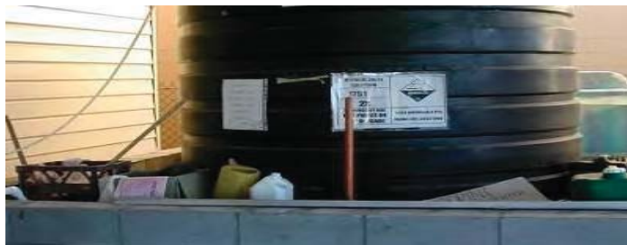
Figure 6 - poor practice where bund contains extraneous material and has not been kept clean and clear.
