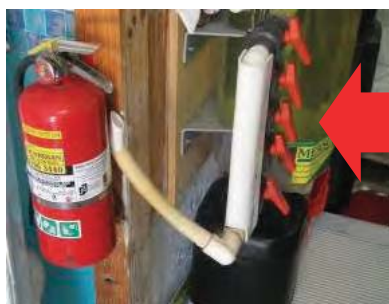
Figure 14 (a) - a fire extinguisher close to a corrosion hazard.
