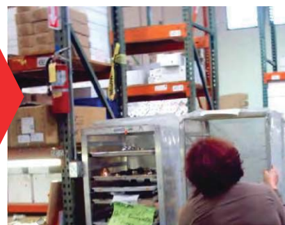
Figure 14 (b) - a fire extinguisher in a difficult to reach position
