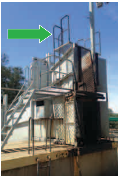
FIGURE 14a Ladder enabling safe access from the ramp to the top of the crate
