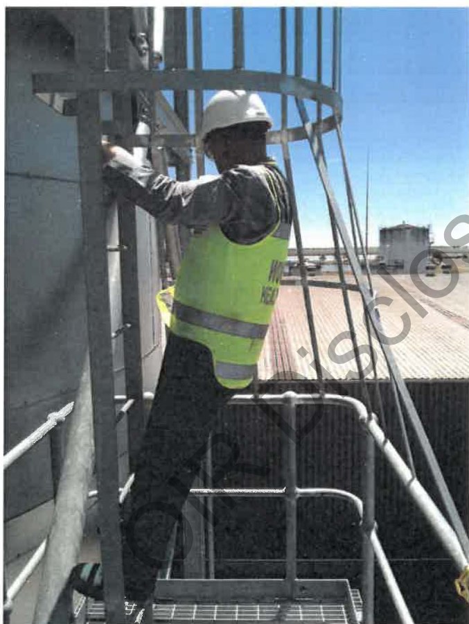
Photograph 2. The bottom of this vertical caged ladder has been flared out and extended down to the top guardrail.
