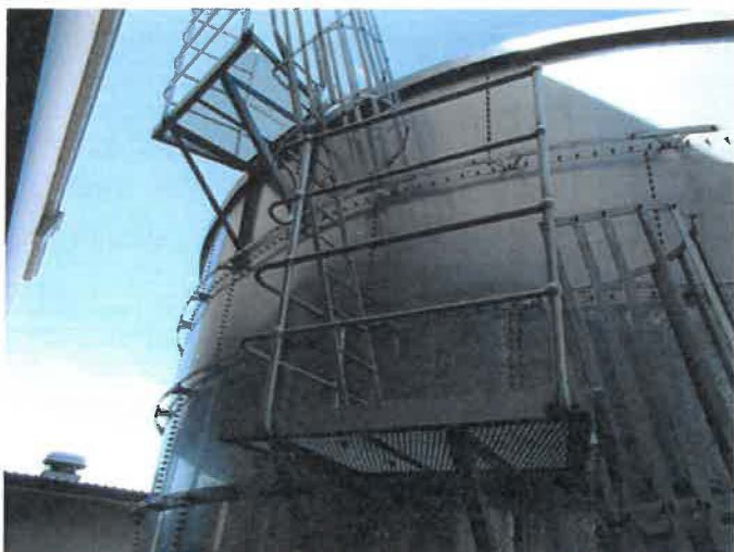
Photograph 1. Inclined caged ladder with additional rails installed to extend the height of the existing top guardrail.
